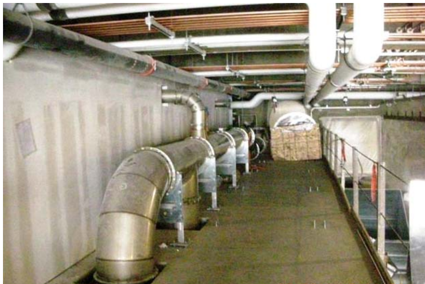
Laboratory level duct work
