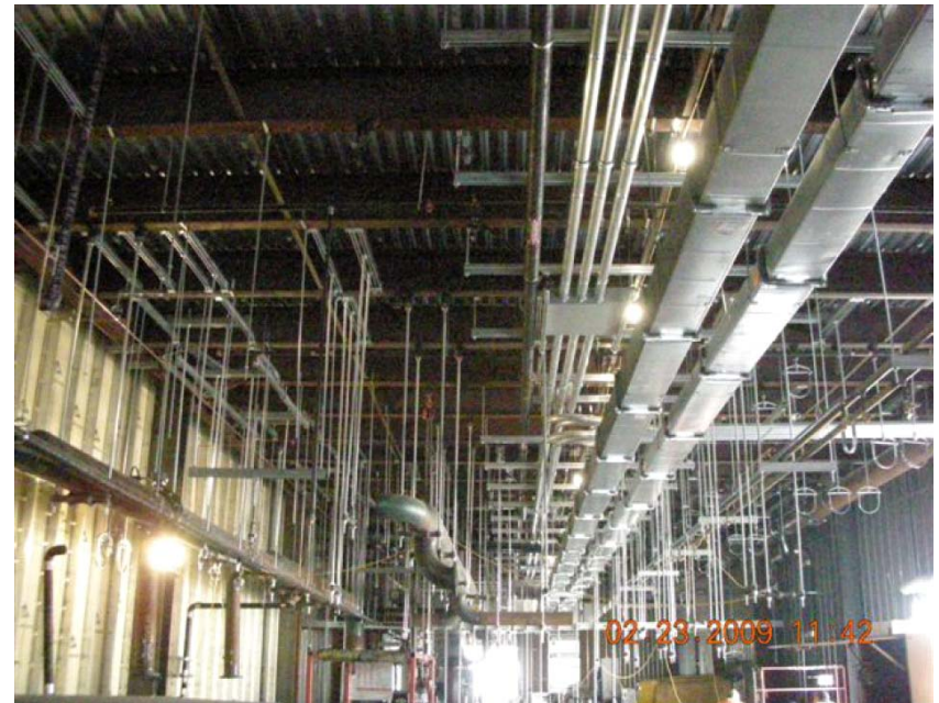
2 nd Floor Central Utility Building – Installation of Duct and Large Bore Pipe
