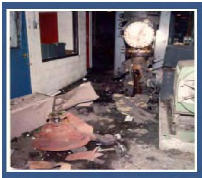
Figure 6 Destruction Caused by Coolant Pump Explosion at the Y-12 Complex in August 1998
