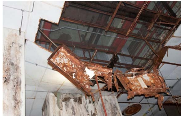
Fig. Y6. Roof/ceiling collapse in Building 9201-05.
