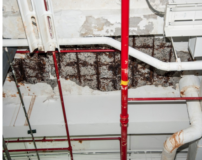
Fig. Y5. Concrete delamination in Building 9204-02.
